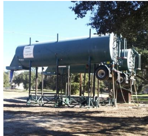
Two storage tanks in RV Park
